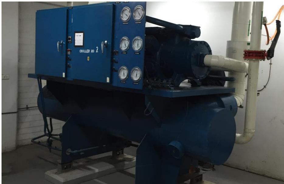
Old Chiller replaced
