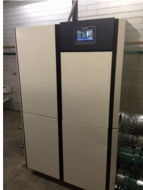
Newly installed Multistack Chiller
